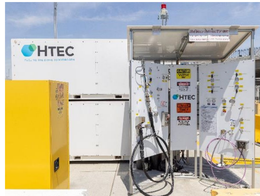
182kg hydrogen storage with dispenser
